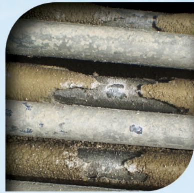
Example of severe scale
