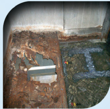
Example of severe corrosion
